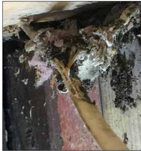
Rodents gnawing on home electrical wiring the cause of nearly 25-percent of "unknown" house fires according to fire-prevention experts.
