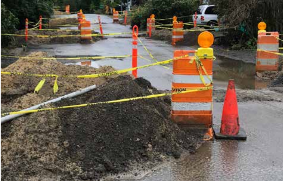
Replacing the connecting collars along the main water lines running beneath 4th Street South and installing water meters is wrapping up for now. The street will be seal-coated later this year when the weather permits.
