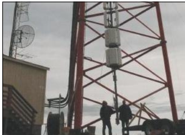
Workers at the new West Lane Translator's 240 foot tower with its panel of twelve antennas located south of Florence
