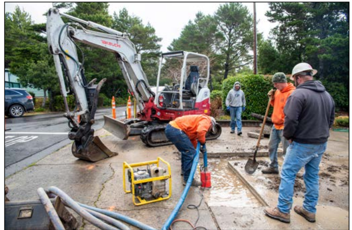
Johnson Rock Products repairing water main on the East side in mid-February.
