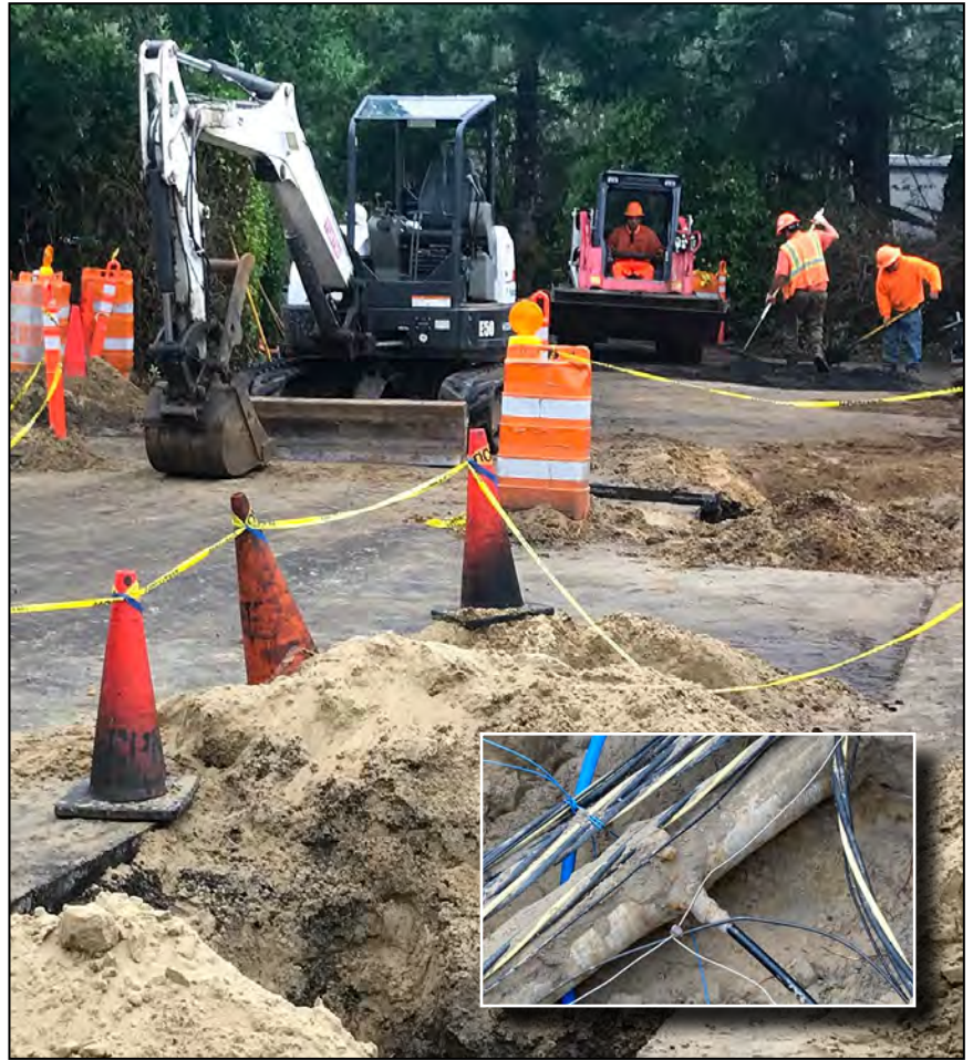
The underground water main repair work by Coast Pavement Maintenance has once again resumed installing the new street-to-residence "T"-couplers that will improve water pressure to the residences served. This month 28 locations along 5th Street are being excavated and upgraded according to GTV General Manager Matt Kennedy. Kennedy says the plan is to replace about 30 lot connections (units) every year.
