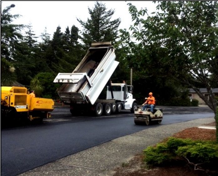
During the month of June, contractor Johnson Stone laid down a new asphalt overlay on the Greentrees clubhouse parking lot
